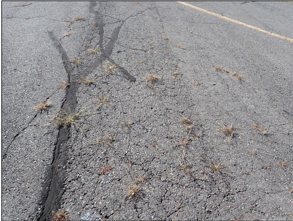
TW-03-20: Alligator Cracking
