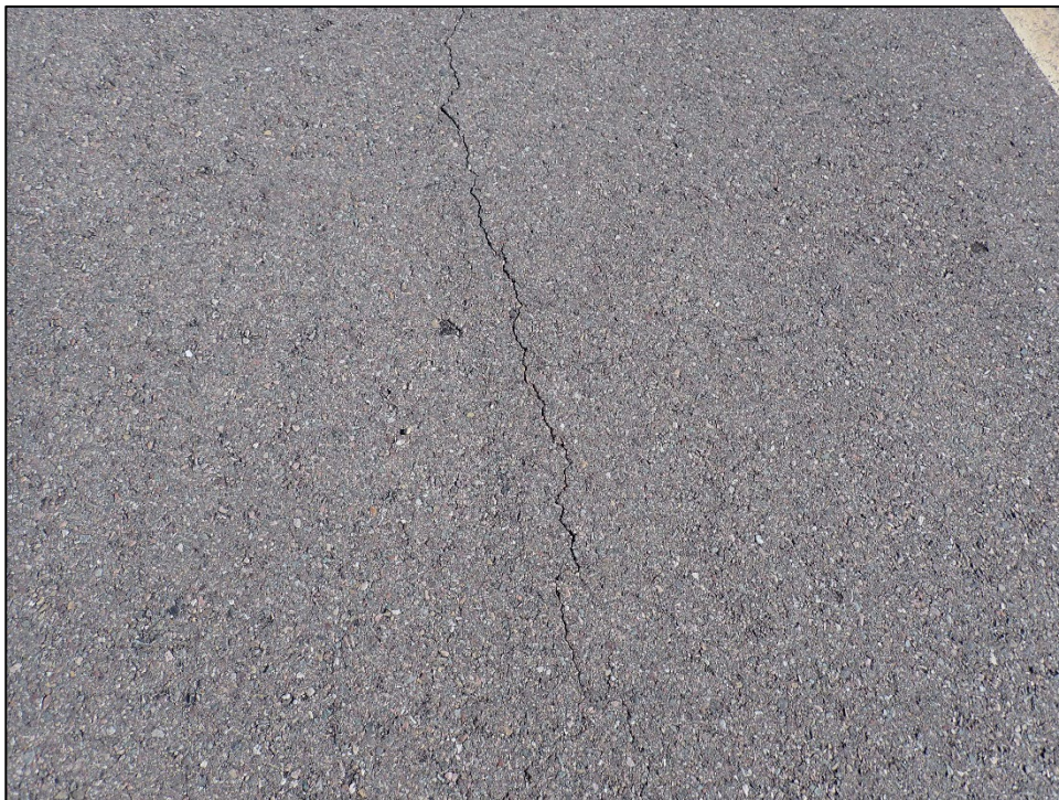
TW-04-02: L&T Cracking
