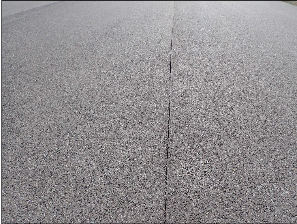
RW12-11-17: L&T Cracking
